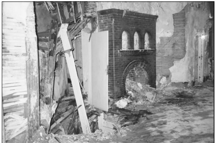
Ongoing water leaks caused serious structural damage in the empty Seminary buildings.
